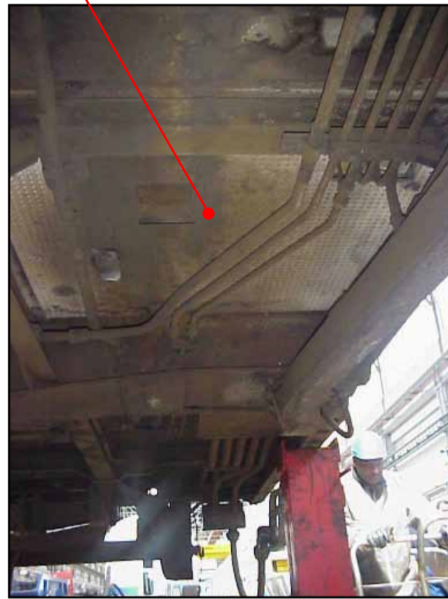
Motor Car 5099 panel to underframe, RHS and LHS Durasteel Panel - Chrysotile and Amosite
