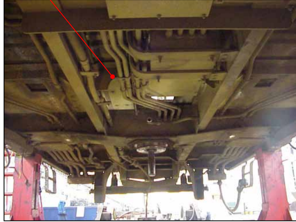
Motor Car 5099 panel to underframe, centre & RHS. Cementitious boarding
